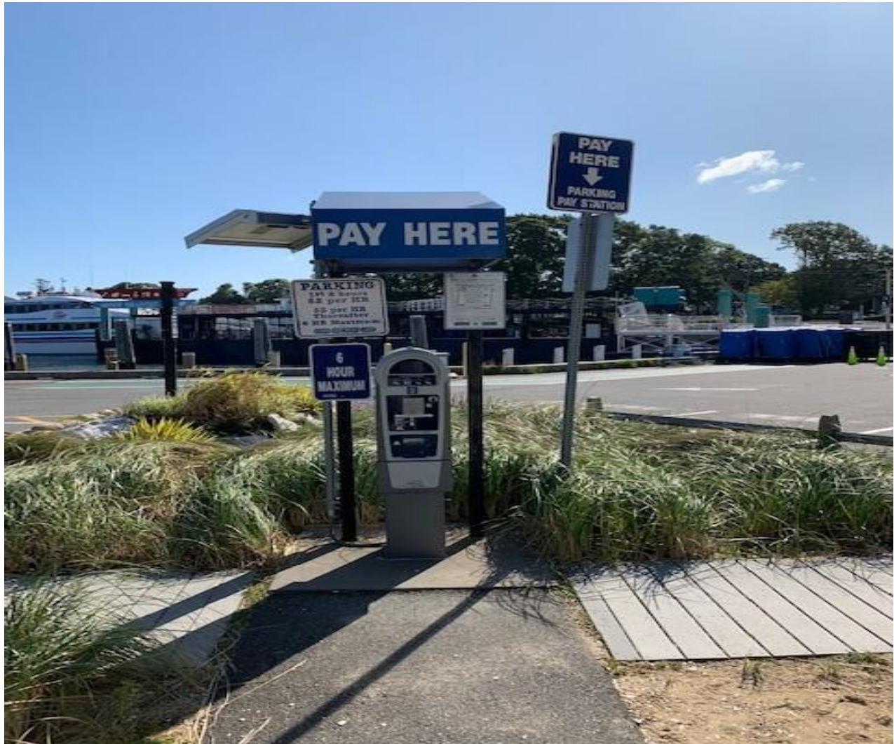
Figure 3 Solar-Powered Parking Pay Station
